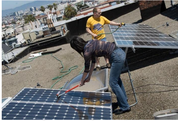
Figure 5: " cleaning the solar panels " (CC BY 2.0) by bkusler
